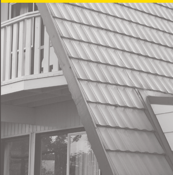
While it looks good from the outside, this rental house has major leaks inside.
