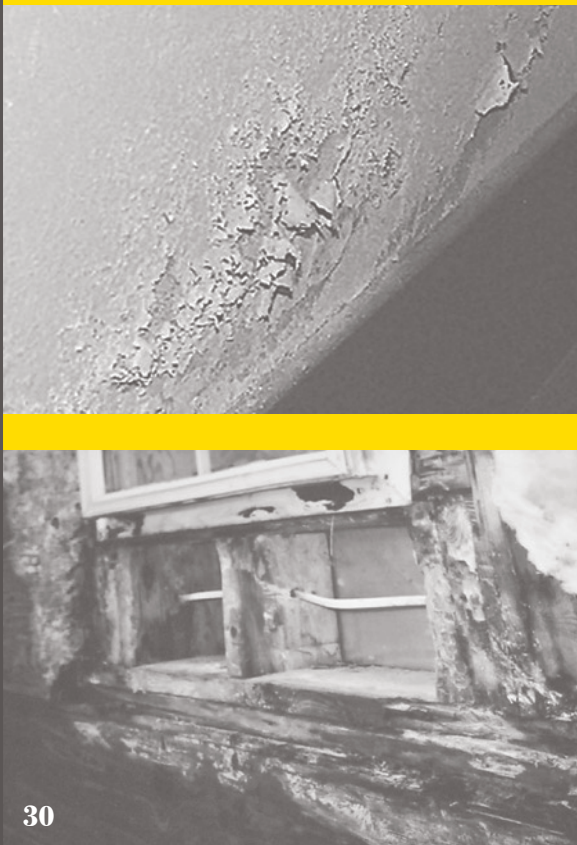
Rising damp and rot. BRANZ photos.
